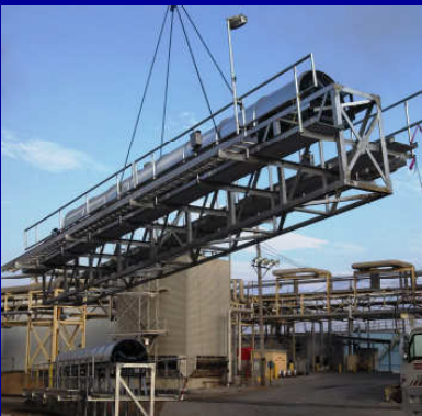
Covered Conveyor Sections
